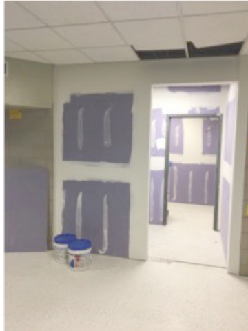
Construction work on the new special education area is well on its way to completion.
